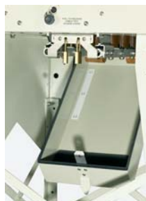
Ring switch earth and test
