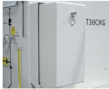
Circuit Breaker Motor
